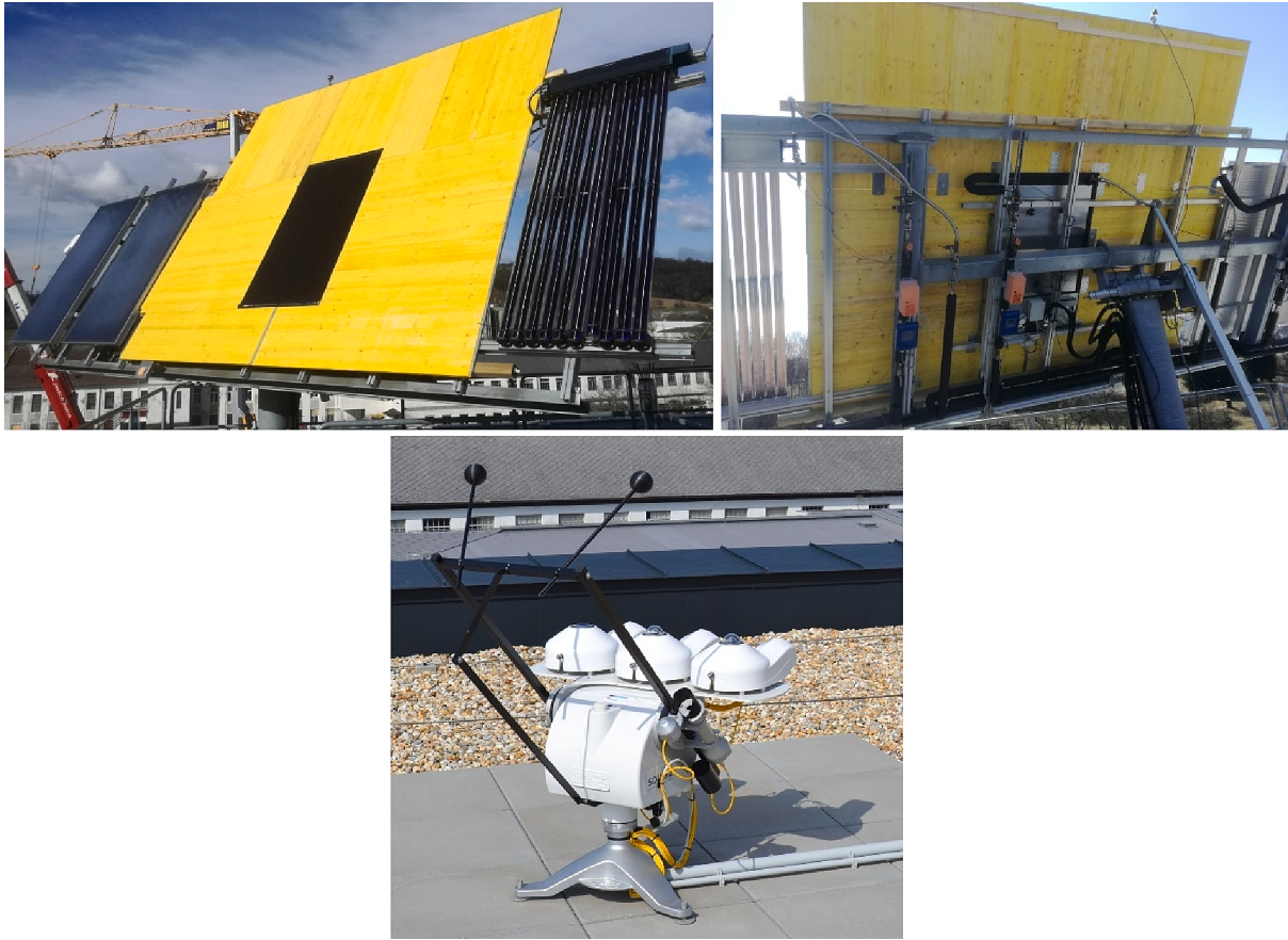
Fig. 2. Photos of the PVT collector test rig: front (above left) and rear (above right) views. Nearby weather station (bottom centre).
